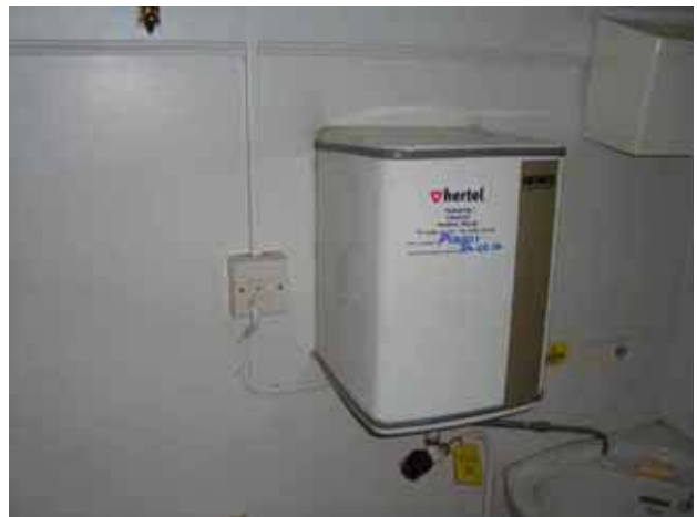
Point of use electric water heater.
