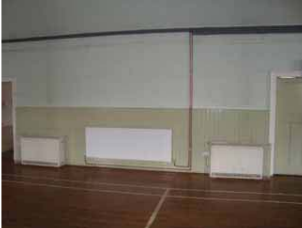
Main Hall indicating electric storage heaters & LTHW radiator.
