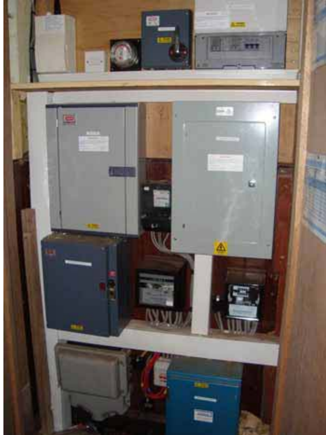
Electrical incoming cable head meters & distribution boards
