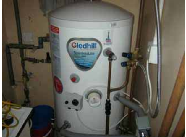
Mains pressure hot water cylinder.
