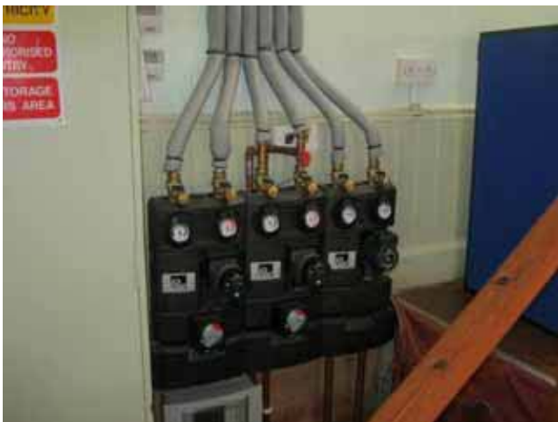
LTHW manifold fed by biomass boiler.
