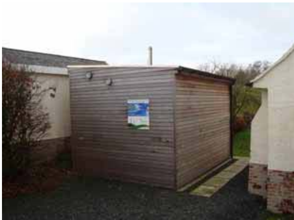
Biomass boiler plant
