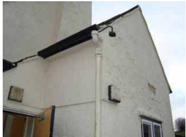
External lighting plus redundant fitting.
