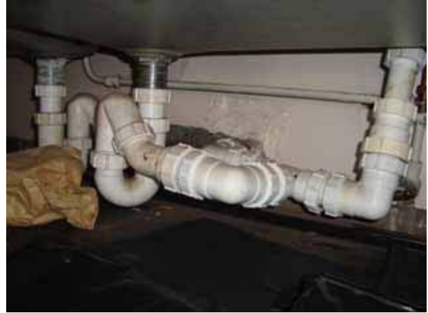
PVC drainage pipework below kitchen sinks.
