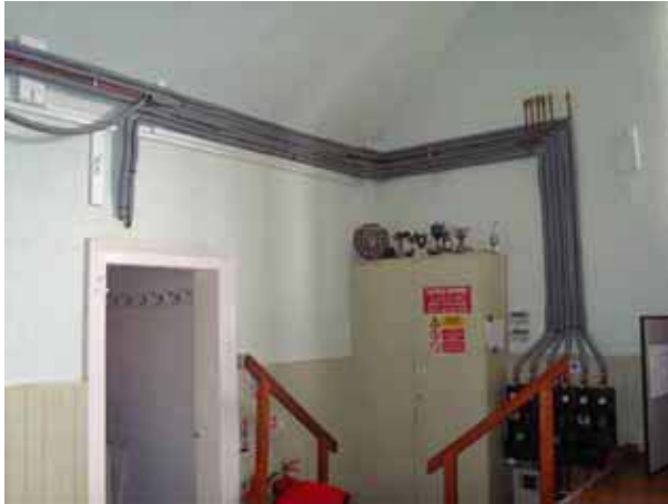
LTHW pipework indicating missing thermal insulation.
